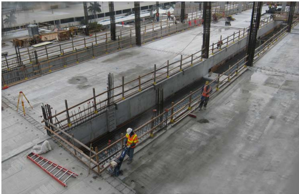
Miami Intermodal Center Construction: Progress Photo February 13, 2009 Rental Car Center (RCC): FM # 249937-5 / MIC-MIA Station: FM # 406800-6 View of MIC-MIA Connector Station Platform Construction
