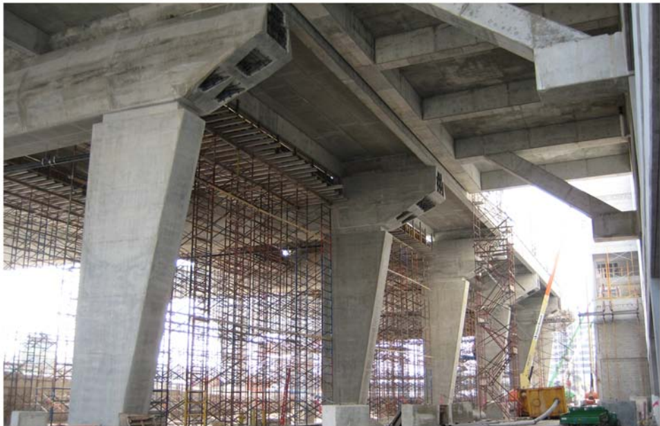
Miami Intermodal Center Construction: Progress Photo February 13, 2009 Rental Car Center (RCC): FM # 249937-5 / MIC-MIA Station: FM # 406800-6 View of underside MIC-MIA Connector Station Platform Construction
