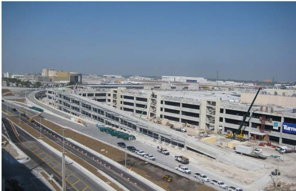
Miami Intermodal Center Construction: Progress Photo February 13, 2009 Rental Car Center (RCC): FM # 249937-5 / MTAR NW 21st Rd: FM # 249937-7 Construction of RCC South Ramp and Improvements to NW 21st Street
