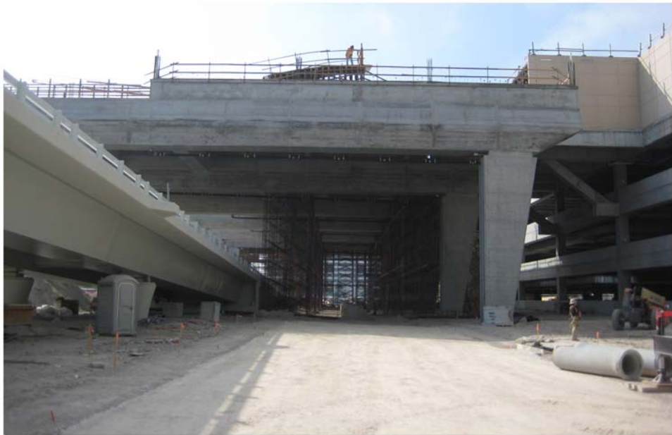
Miami Intermodal Center Construction: Progress Photo February 13, 2009 Rental Car Center (RCC): FM # 249937-5 / MIC-MIA Station: FM # 406800-6 / MTAR: FM # 249937-4 View of Ramp "C" and Straddle Bent Construction
