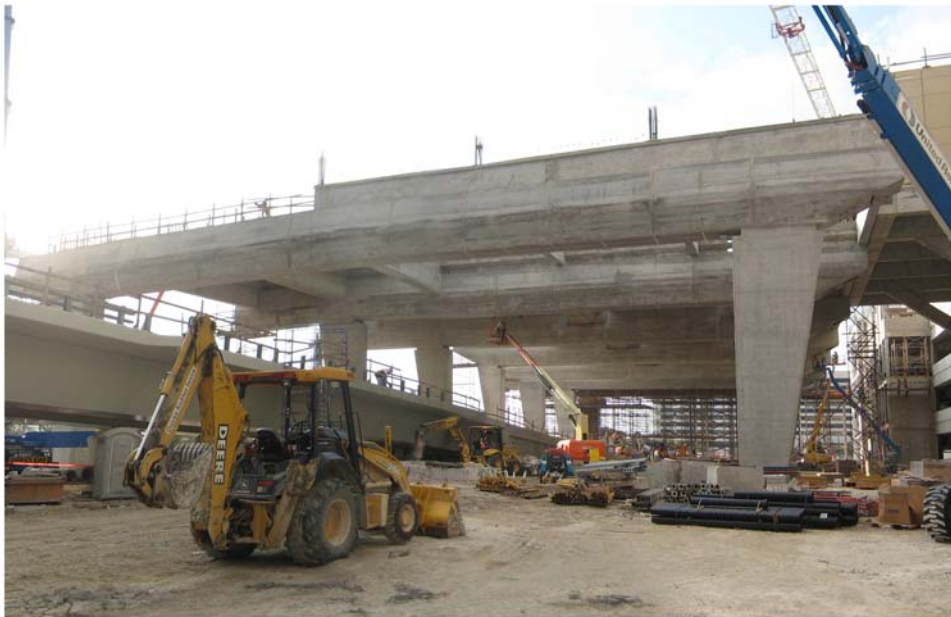
Miami Intermodal Center Construction: Progress Photo January 27, 2009 Rental Car Center (RCC): FM # 249937-5 / MIC-MIA Station: FM # 406800-6 / MTAR: FM # 249937-4 View of Ramp "C" and Straddle Bent Construction
