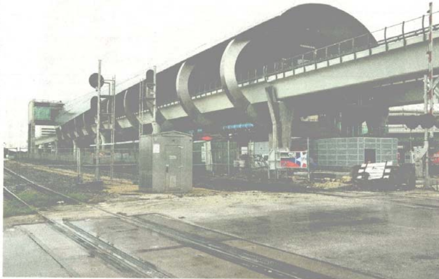
The new Metrorail Airport Station nears completion. Tri-Rail tracks run parallel to the Metrorail route.
