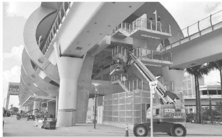
Work continues at the Metrorail and Metrobus station component of now-rising Miami Central Station.
